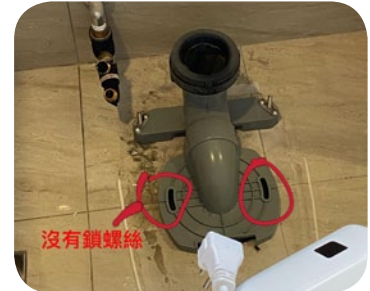
Detection of incomplete sealing--shortage of 2 sets of fixing screws.
