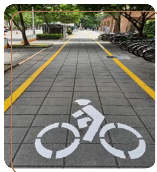
Planning and installation of pavement signs and markings at the car park of Prince House Shuiyuan
