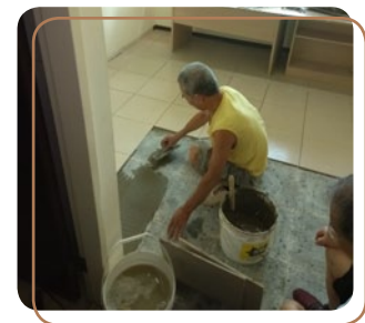
Replacement of lifting floor tiles at Room A305 at Prince House Changxing.
