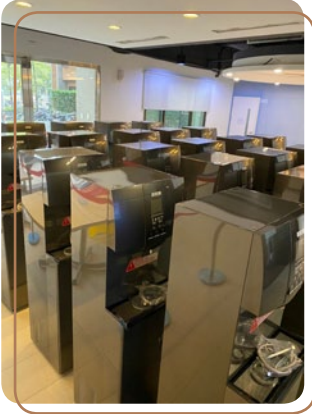
Water dispenser replacement at Blocks B and C of Prince House Shuiyuan.
