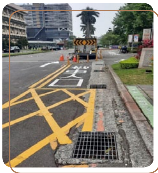
Planning and installation of lane signs and markings at the car park of Prince House Shuiyuan
