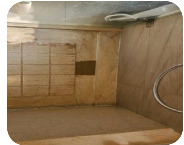
Detection of water seal problems in all drainage systems
