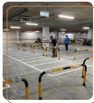
Upgrading of the inverted U-shaped guardrail at the car park of Prince House Shuiyuan
