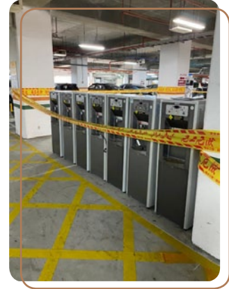
Water dispenser replacement at Block A of Prince House Shuiyuan and Block D of Hsiu Chi House.
