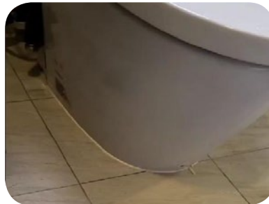
Validation of odor from the toilet bowl. Removal of the toilet bowl
