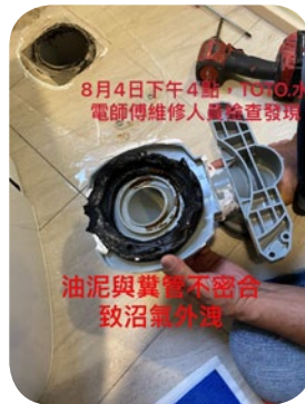
Alignment failure of the wax ring and floor flange, leading to poor sealing.
