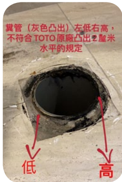
Insufficient floor flange height leading to poor sealing.
