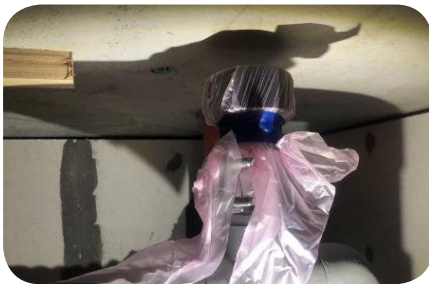
Verification of air valve problems
