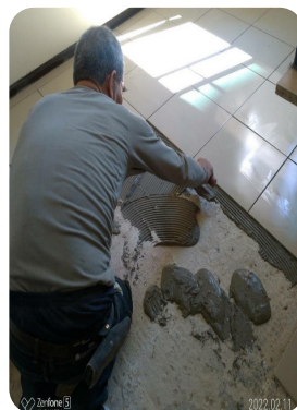
▲ Replacement of lifting floor tiles in Room A232 of Prince House Shuiyuan.
