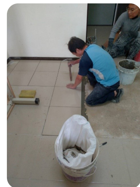
▲ Replacement of lifting floor tiles in Room A252 of Prince House Shuiyuan.
