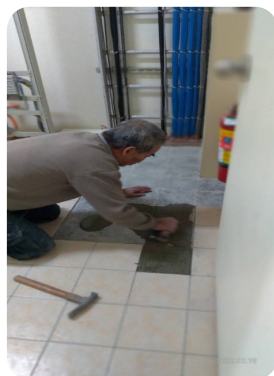
▲ Replacement of lifting floor tiles of the electrical room in Zone B, 5F, Block A, Prince House Changxing.
