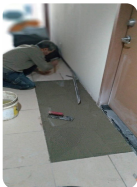
▲ Replacement of lifting floor tiles in Room A1140 of Prince House Changxing.
